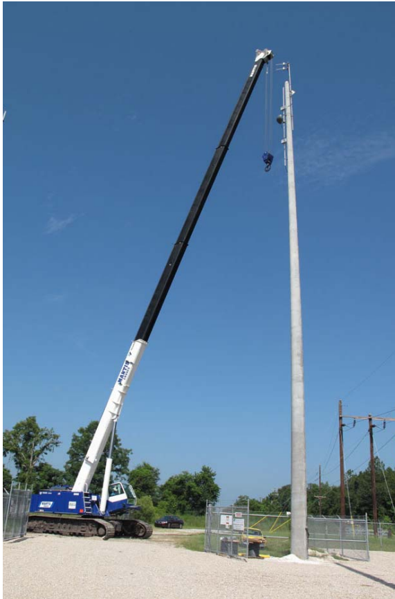
Tadano Mantis 15010 after setting the final pole in a seven mile powerline installation.
